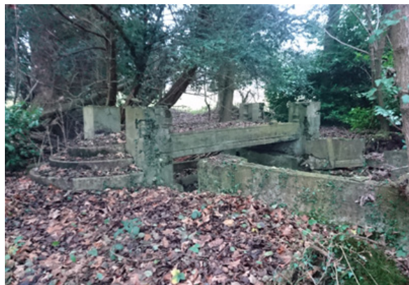
Derelict stonework from the lido complex
