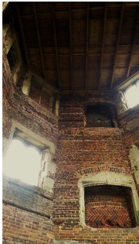
Interior view of the main Tower showing the failing roof
